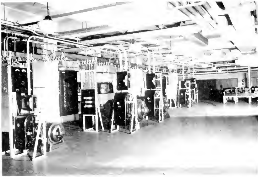
THE POWER ROOM OF THE WASHINGTON, D. C., DISTRICT-METROPOLITAN-NATIONAL DIST. OFFICES, SHOWING CHARGING MACHINES IN THE FOREGROUND AND RINGING MACHINES IN THE RIGHT BACKGROUND.
